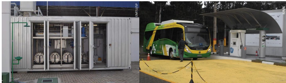
Hydrogen production and refueling station
