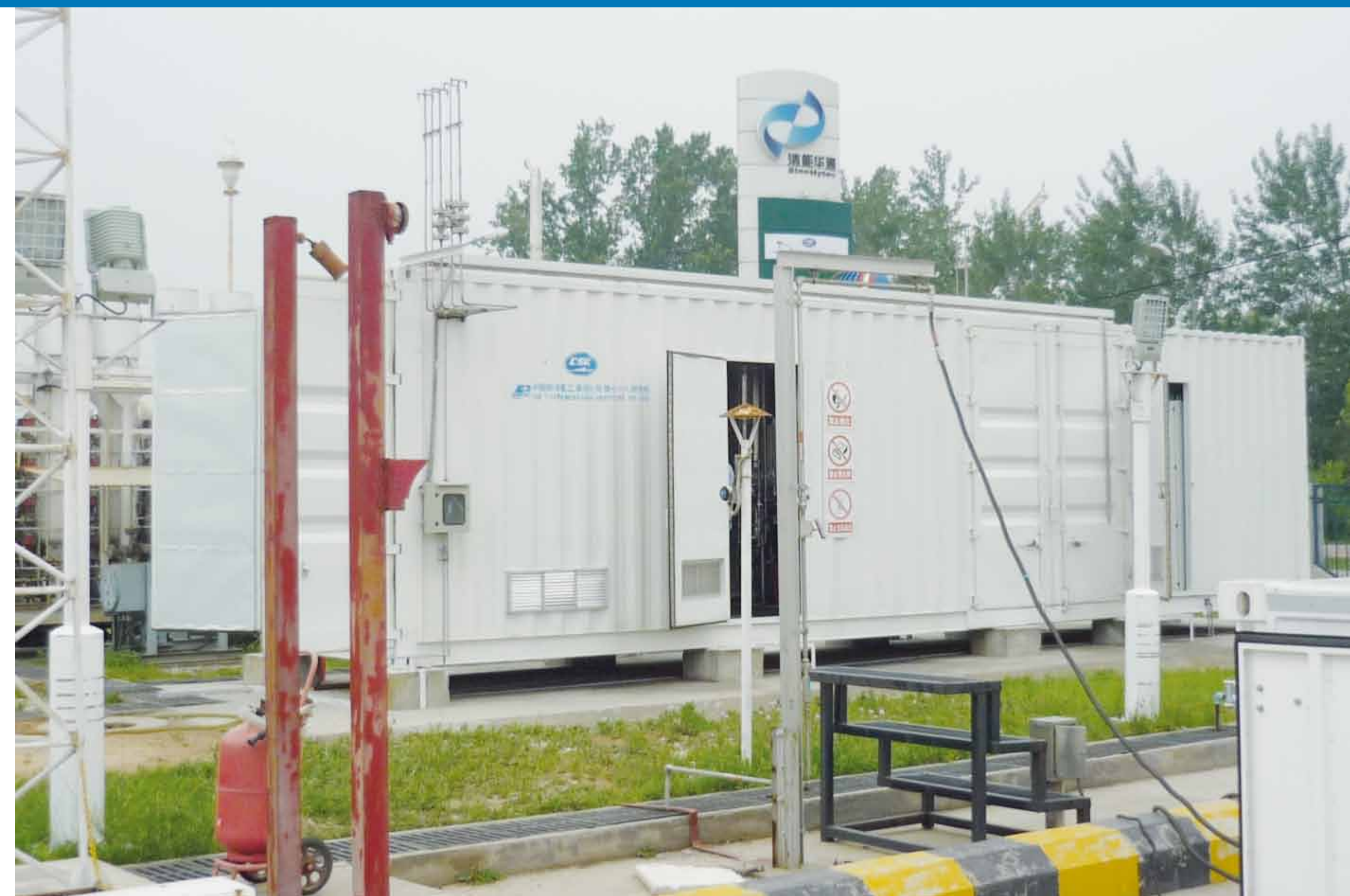
The first skid container type 50Nm 3 /hH 2 electrolyser in China
