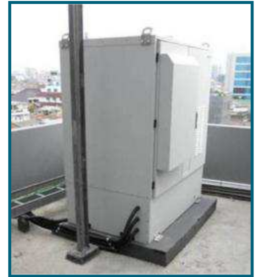
Rooftop installation of Ballard ElectraGen™-ME fuel cell system in Indonesia
