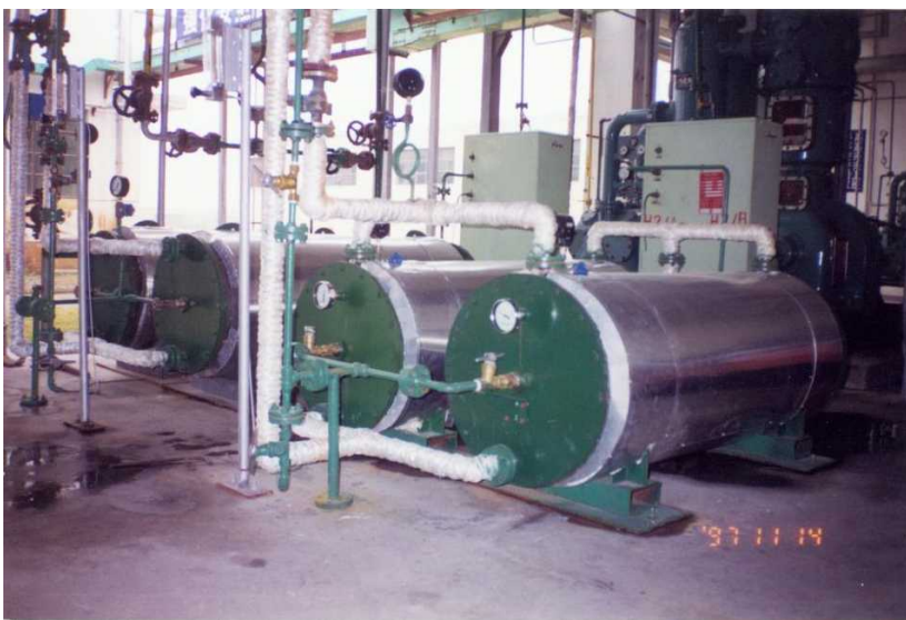
MH hydrogen storage units for hydrogen recovery and purification
