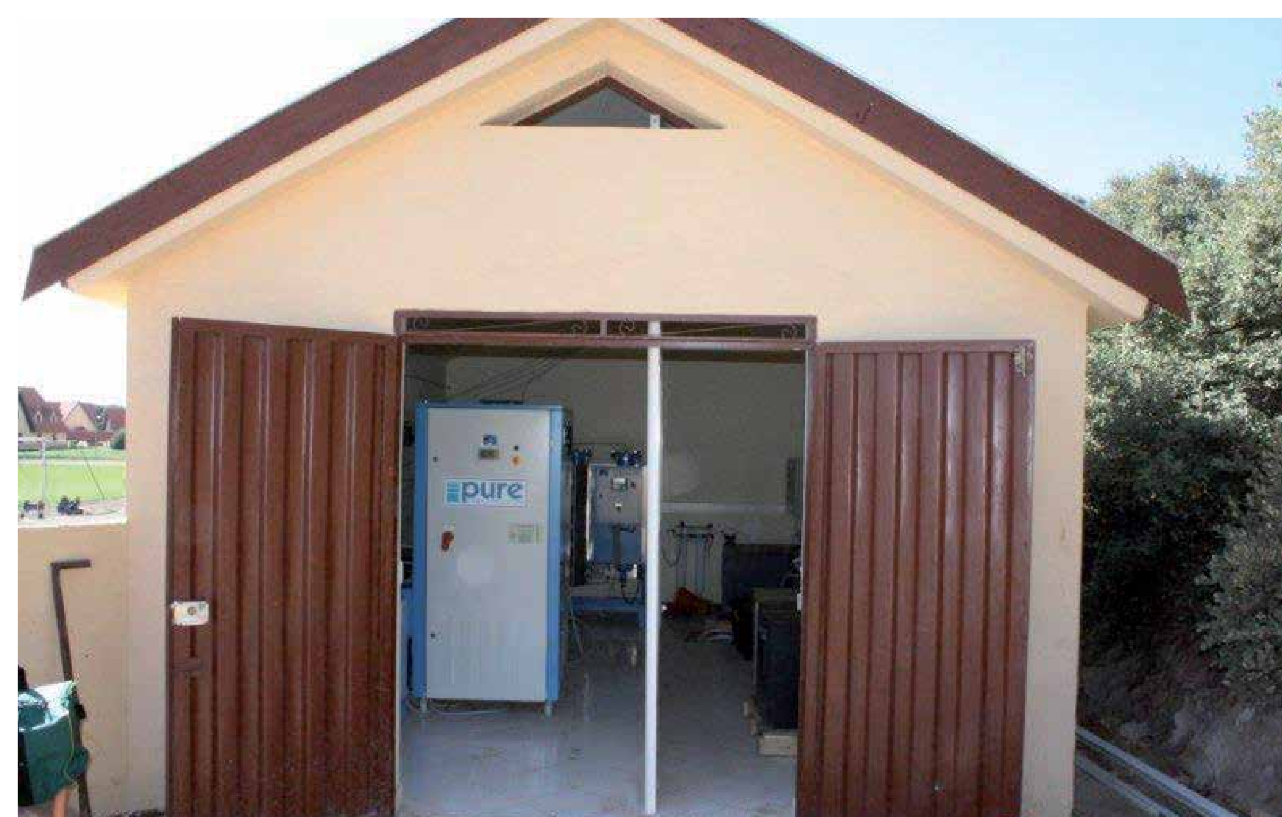
Hydrogen equipment within plant room
