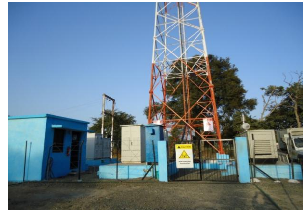
Fuel Cell system as power back up for telecom tower
