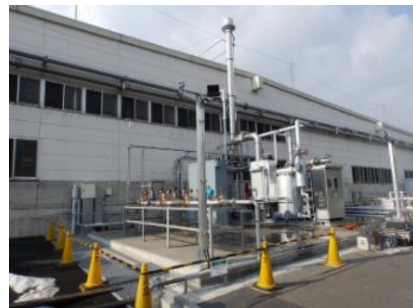
Hydrogen Boiler - 24 hours operation
