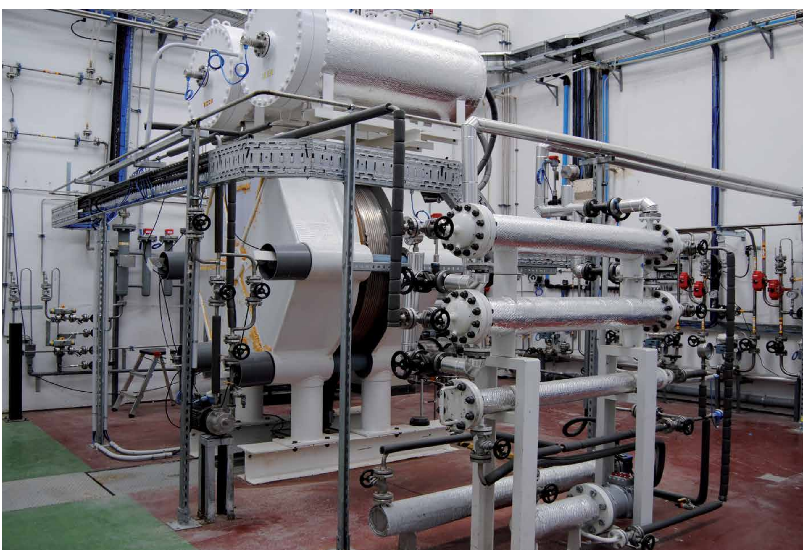
IHT Electrolyser – Hydrogen Foundation Aragon facilities
