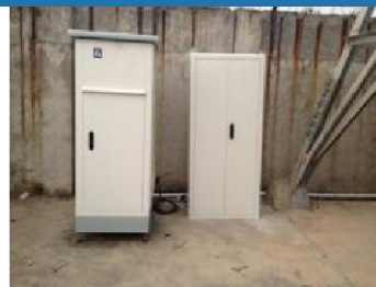
联通厦门基站 China Unicom Base Station in Xiamen
