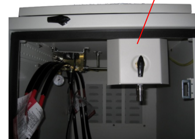
In-cabinet ground sites
