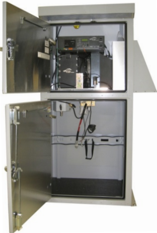
2.5 kW Railroad Backup
