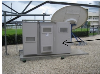
Before with Battery Cabinet
