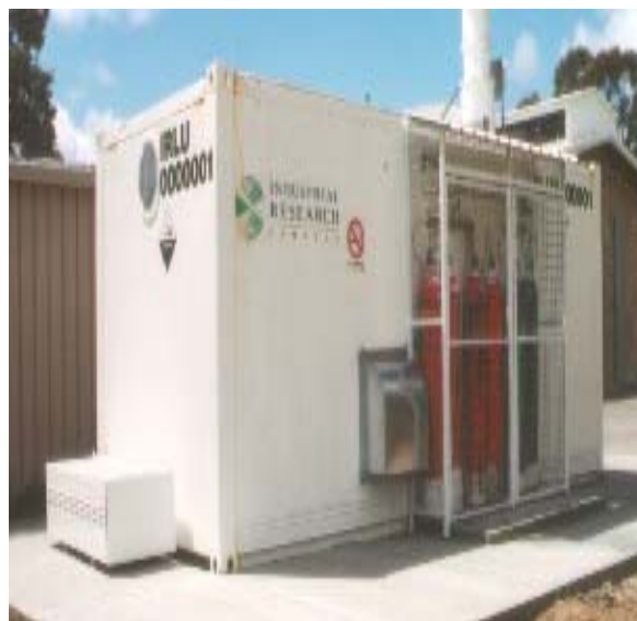
The 6 kW alkaline fuel cell system installed and commissioned at Murdoch University, Western Australia
